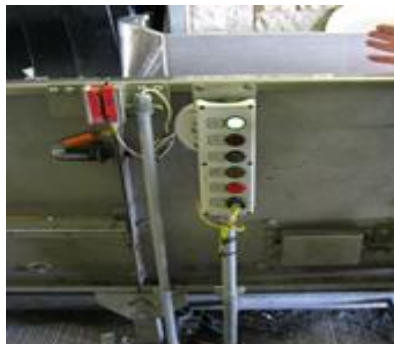
REMOTE (EXTERNAL) OPERATOR CONTROL STATION
