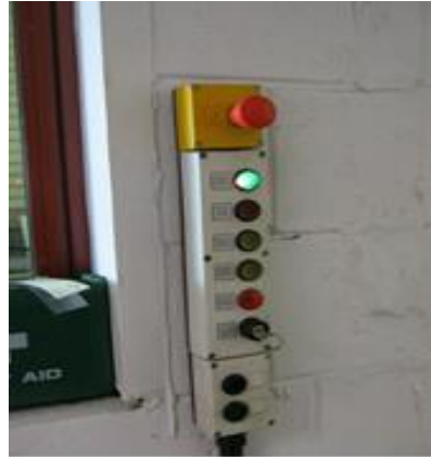
REMOTE (INTERNAL) OPERATOR CONTROL STATION
