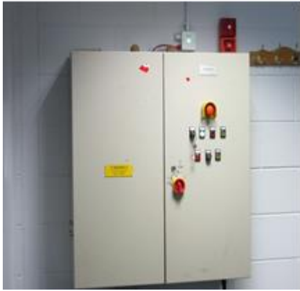
MAIN CONTROL PANEL (WALL MOUNTED) COMPLETE WITH MAIN SYSTEM ISOLATOR
